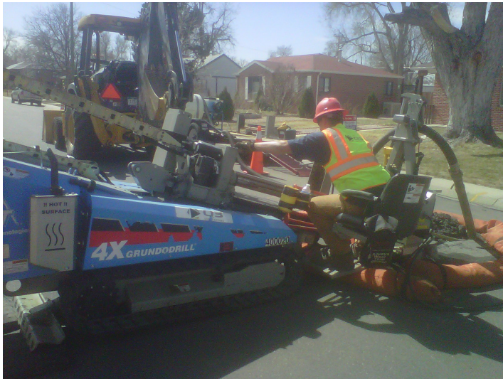
For Q3, one of the biggest benefits of the compact drill on utility projects is the ability to operate in tight working conditions.
