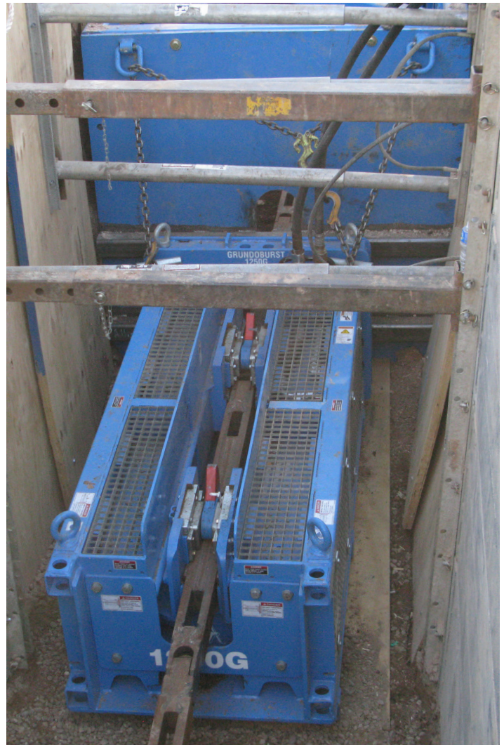
A Grundoburst 1250G static pipe bursting unit from trenchless equipment manufacturer TT Technologies, Aurora, Ill., was used as the pulling unit for the Amarillo, TX project.
