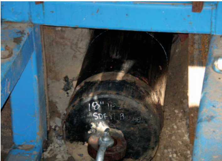
This image shows the 18-inch HDPE being pulled into the extraction cage after another productive, successful slipline.
