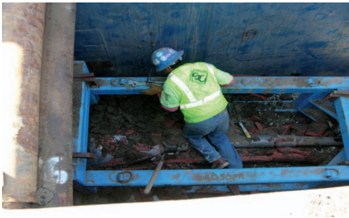
The pipebursting head with new 18-inch HDPE is being pulled into extraction cage.
