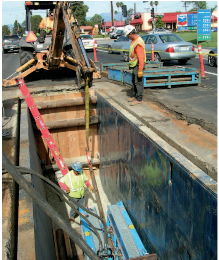
Crews utilized a Grundoburst Static Pipebursting system with Quicklock rods, bursting 15-inch VCP and pulling in 18inch HDPE in this image.
