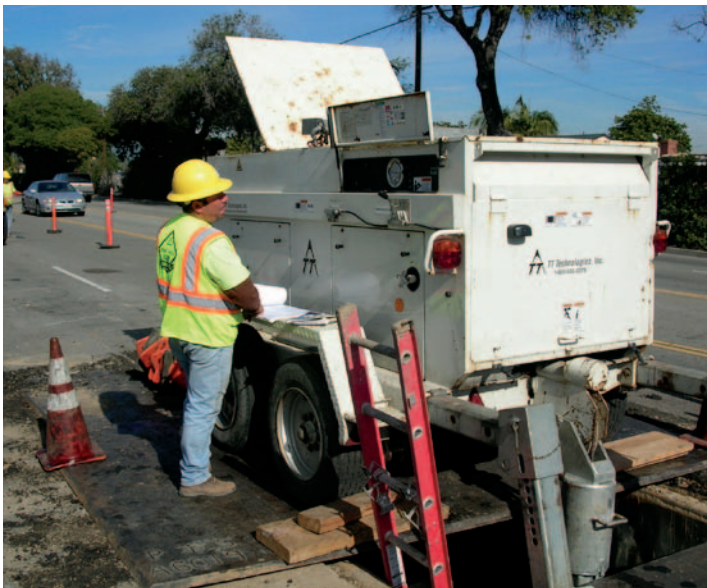
Crews used a 20-ton, constant tension Grundowinch for sliplining the 18- and 22-inch pipes.
