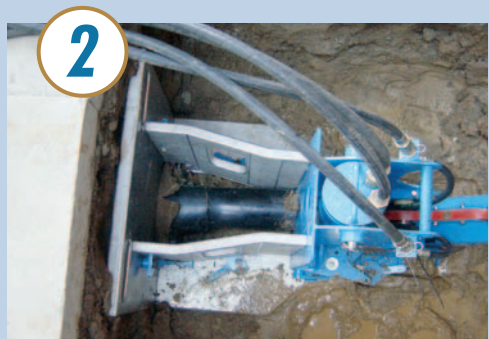
Once the launch and exit pits are prepared, the GRUNDOTUGGER unit is placed in the exit pit and connected to a hydraulic power pack.
