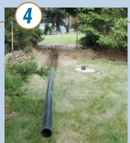
The GRUNDOTUGGER unit pulls winch line, the bursting head and new pipe through the existing lateral. This bursts the old lateral, forcing the fragments into the surrounding soil while pulling in the new pipe.
