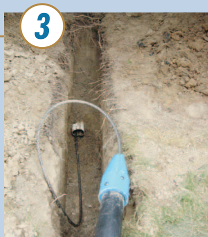
At the launch pit, the winch cable is rodded through the existing line to the exit pit. The bursting head is attached to the new pipe and connected to the winch line.
